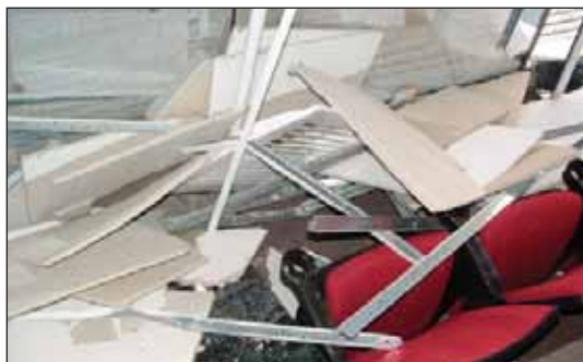
Portions of entire ceilings crashed down, affecting the internal fire protection structure even further.
